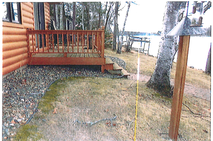
Lakeside deck, cedar construction, built in 2008, significant deterioration
