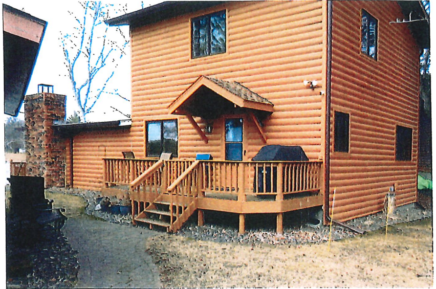
Front deck, cedar construction, built in 2008, significant deterioration
